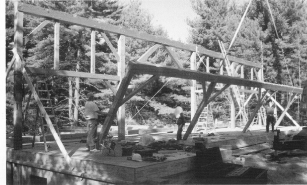
In this frame, of recycled fir, we were fortunate to have very long timbers available for the plates. Had that not been the case, scarf joints would have been required.
